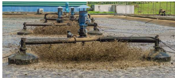
Activated Sludge Treatment 2
