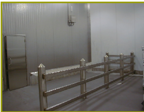
Courtesy AMI Facility Design Task Force
