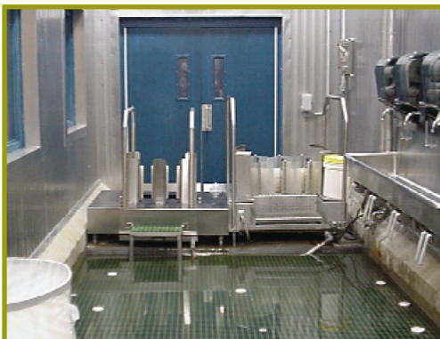
Courtesy AMI Facility Design Task Force
