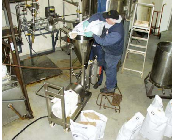
At a flavors manufacturing plant, this inline SLIM mixer is wheeled between several 1,000-gallon vessels to make different gum dispersions.
